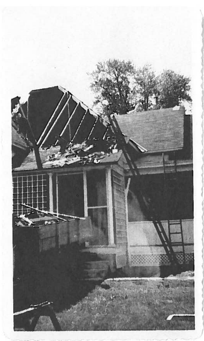
East side of the house during the repair process after the fire. Shows fire debris from the attic being load from above the screened in porch south of the rear door of the home.
