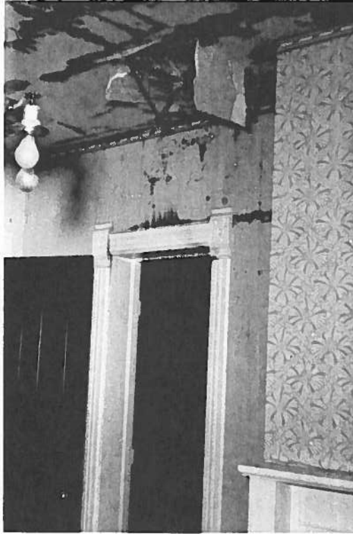
East wall of the living room. Fire place on right and doorway Into a bedroom east of the living room.
