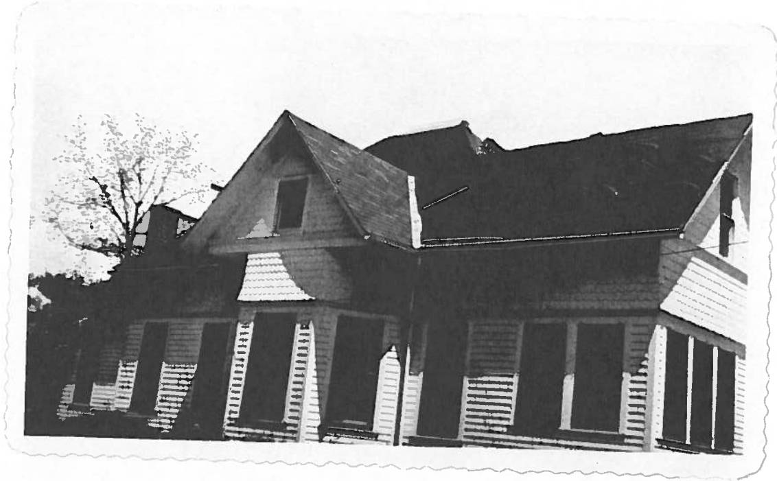
West side of the house during the repair process after the fire.
